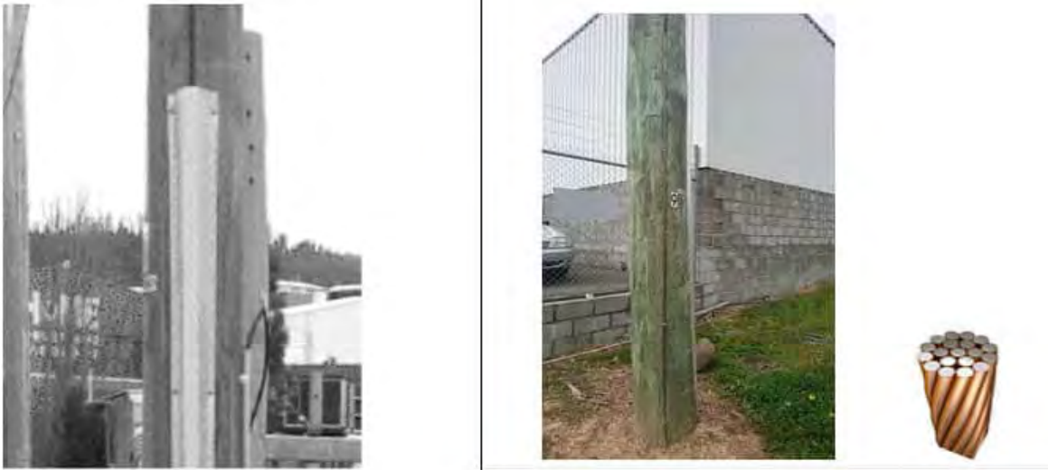
Figure 3: Pole earth copper theft is resisted by steel covers or using copper clad steel
