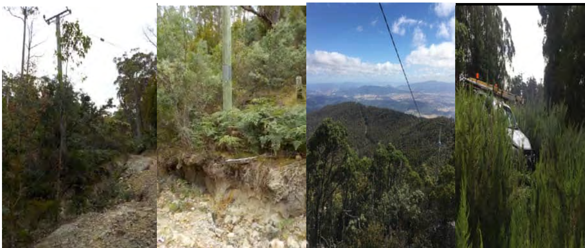
Figure 28 Examples of high slope access tracks & track washout near pole footing
