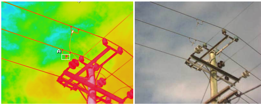
Figure 27: A Live Line Clamp through a thermal imaging camera and a normal camera
