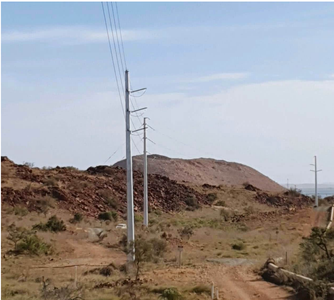
Photo 1 – Example Transmission Poles
