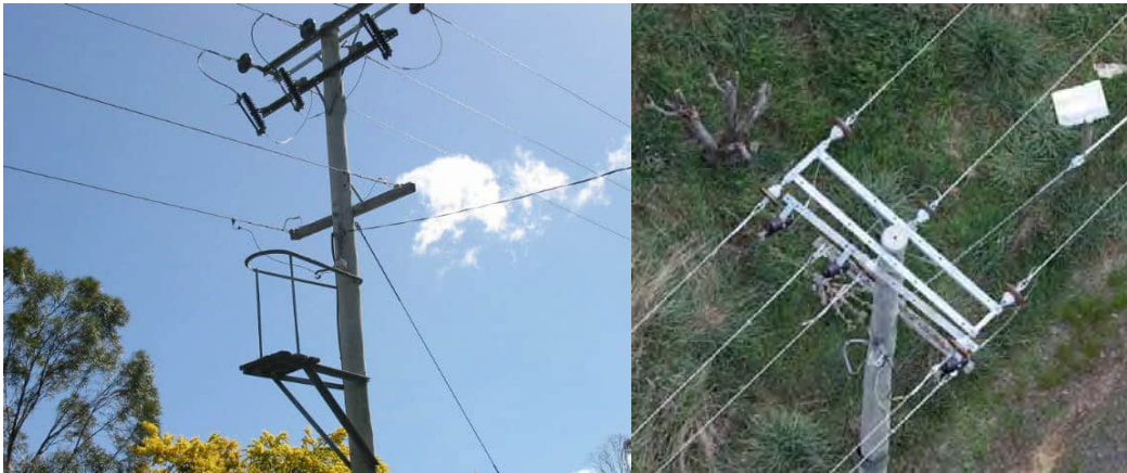
Figure 24: The same pole as seen from the ground and from the air
