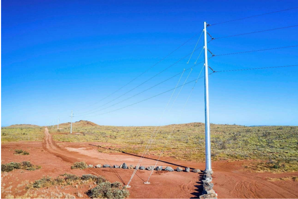
Photo 2 – Example Transmission Poles
