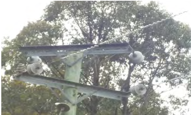
Figure 11: Three in series HV spiral dampers per conductor on a long span
