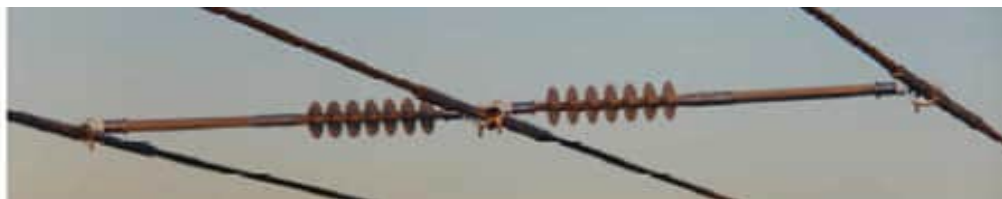
Figure 30 shows a HV mid span spacer set for AAC damping galloping solution
