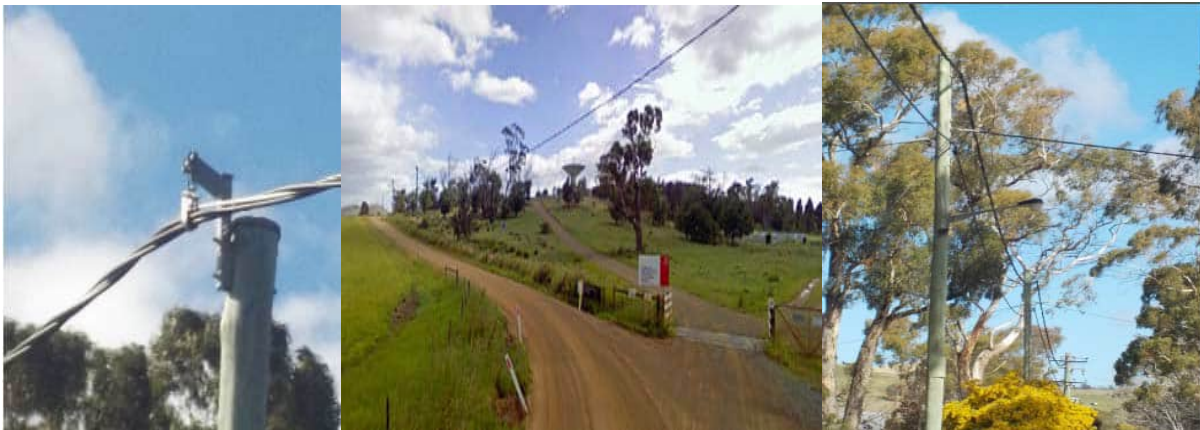
Figure 32 existing non-metallic screened (NMS) HV ABC conductor
