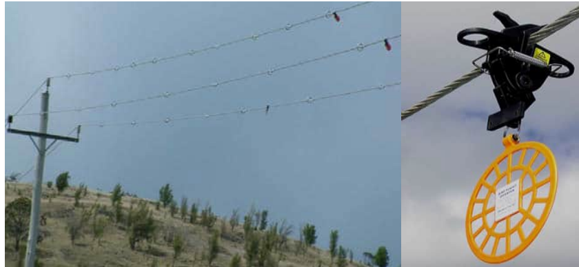
Figure 8: Bird diverters installed on conductor (but not on substandard conductors)
