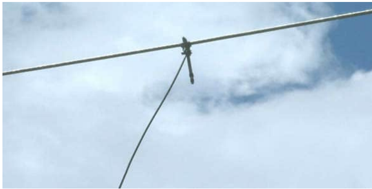
Figure 9: Live line clamp directly connected
