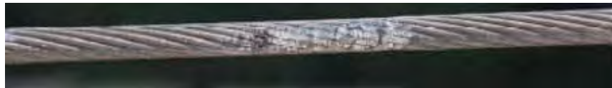
Figure 29 shows one of two adjacent AAC midspan conductor arc melts from galloping
