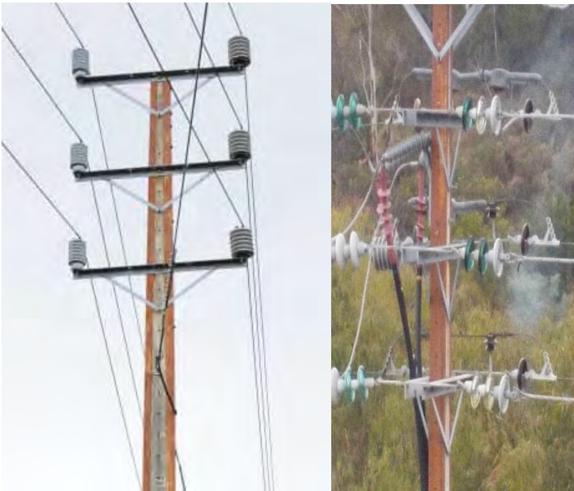
Figure 4: Steel HV cross arms and insulators on dual circuit 33kV and 33 kV and 11kV circuits on a stobie pole
