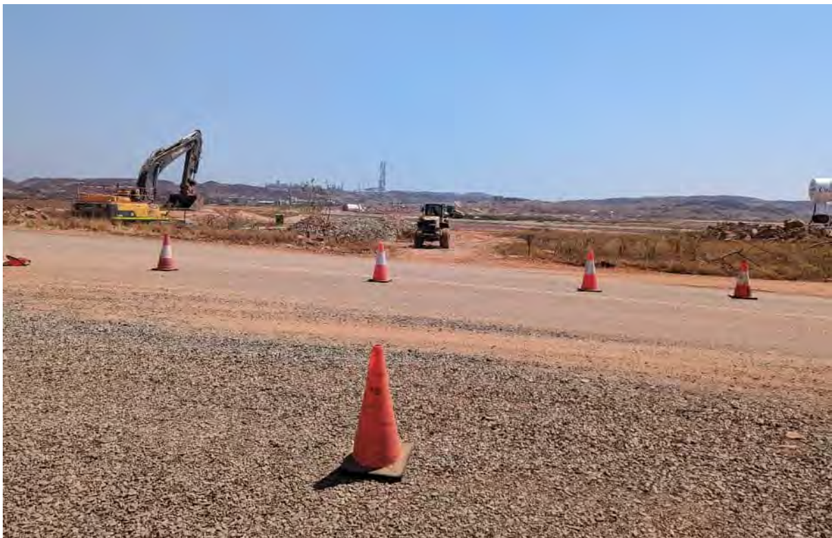
Photo 6 - Current construction and clearing works commenced at the tidal inlet area associated with the Perdaman Urea project and road upgrade (Photo taken 9th October 2023)
