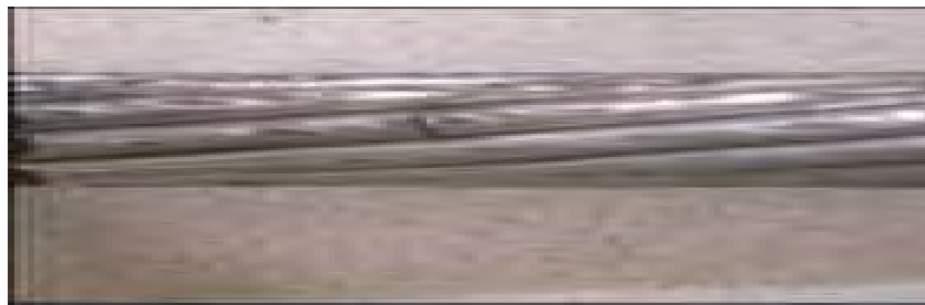
Figure 22 shows example of fretting conductor fatigue failure risk in AA or ACSR conductor
