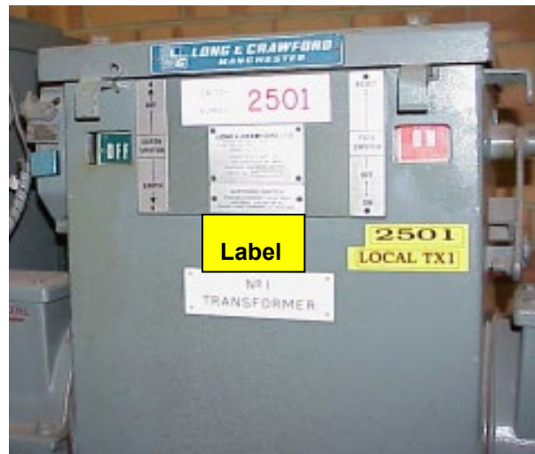
Figure 15 – ‘Long & Crawford’ RMU label location.
