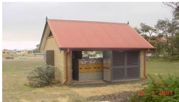
Figure 3 – Brick enclosure Substation.
