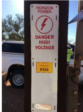
Figure 41 – Warning label for poles with high voltage.
