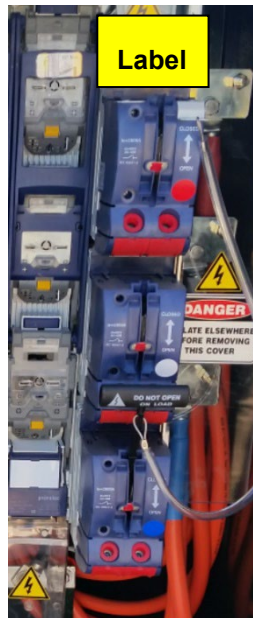
Figure 22 – ‘Pronutec’ LV Disconnecter label location.
