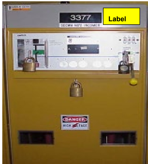
Figure 14 – ‘Merlin Gerin’ RMU label location.
