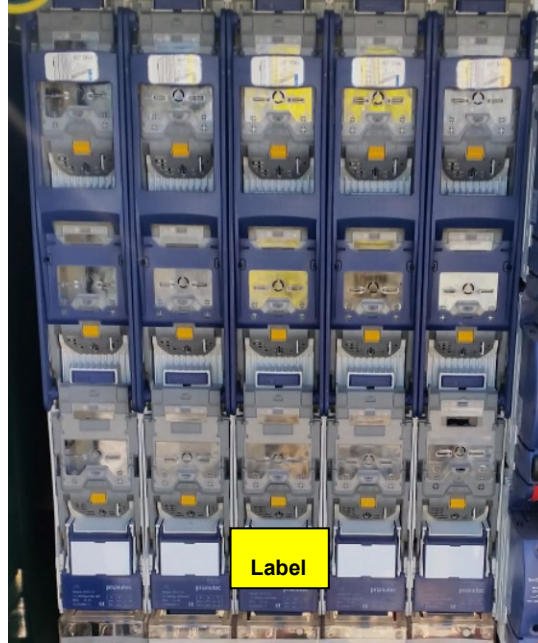
Figure 27 – ‘Pronutec’ Fuse Switch label location.
