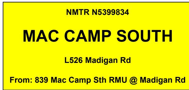
Figure 6 – Metering Transformer label example.
