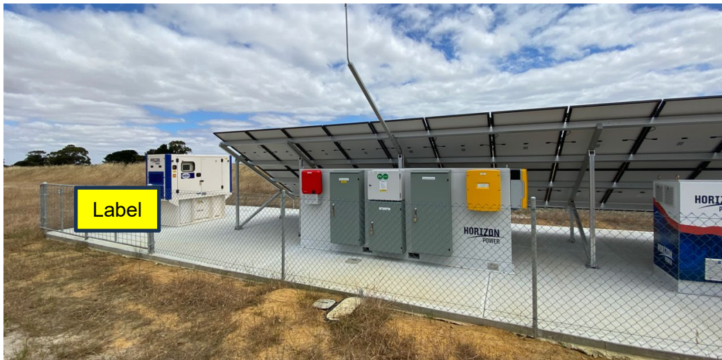
Figure 61 – Typical Standalone Power System (SPS) site label location.
